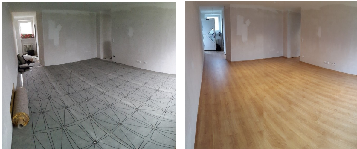
Figure 2 Installation of the SensFloor® underlay and same view after installation of the laminate
